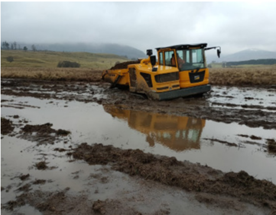
Figure 18: Ground conditions at Laird's Haugh, Rottal Estate in January 2026 were unsuitable for construction and figure 18 shows heavy plant being unable to move across waterlogged areas of the site.
