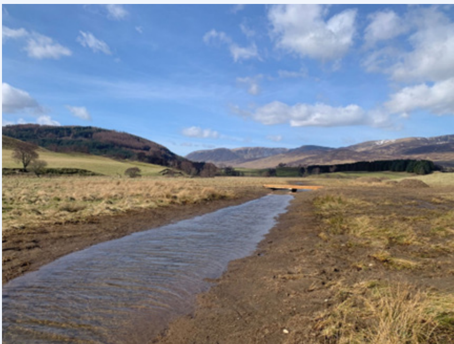
Figure 8: The completed Laird's Haugh wetland high-stage offtake and vehicle access bridge is shown in figure eight.
