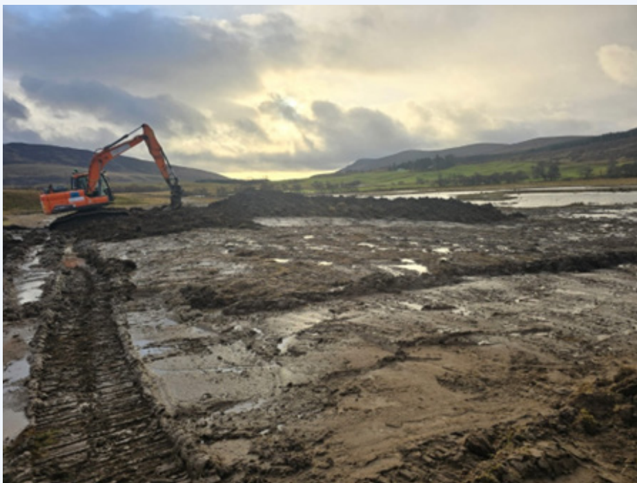
Figure 6: A digger on-site at Adielinn excavating the southern end of the offtake channel, where it meets the scrape cluster is shown in figure six.
