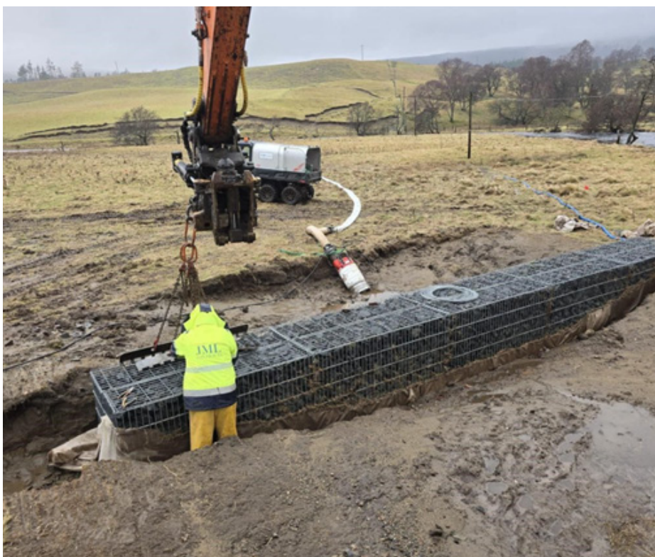
Figure 5: Adielinn fish gabion barrier is shown being installed Laird's Haugh in late 2025 in figure five.
