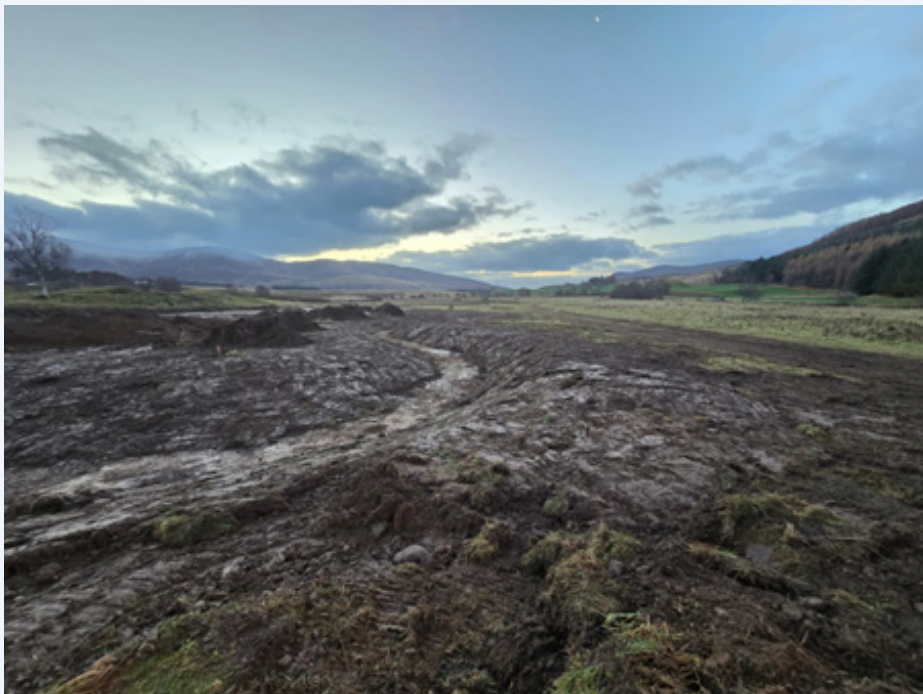
Figure 5: Construction at Adielinn commenced in October 2025. Figure five shows the Adielinn high-stage offtake under construction looking south-east.
