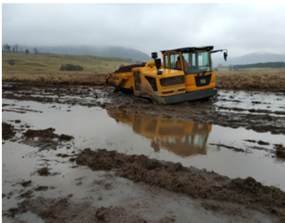
Figure 18: Ground conditions at Laird's Haugh, Rottal Estate in January 2026 were unsuitable for construction and figure 18 shows heavy plant being unable to move across waterlogged areas of the site.
