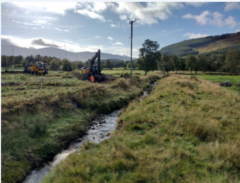
Figure 1: Construction phase began on site at March Burn in September 2025. Figure one shows a digger onsite prior to excavation of the original channel.
