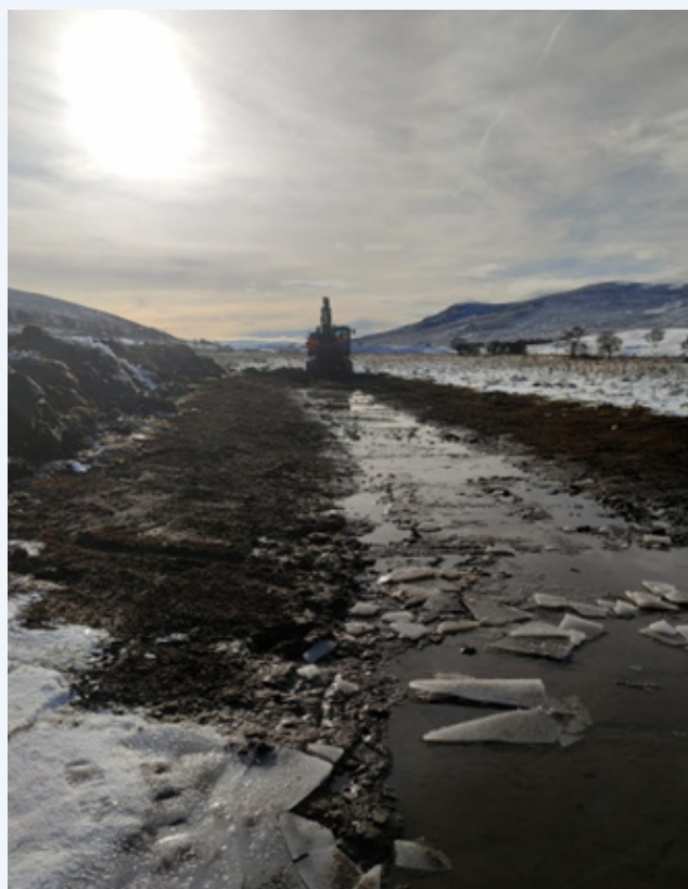
Figure 11: Construction at Laird's Haugh commenced in January 2026. Figure 11 shows a digger constructing the Laird's Haugh high-stage offtake in February 2026.
